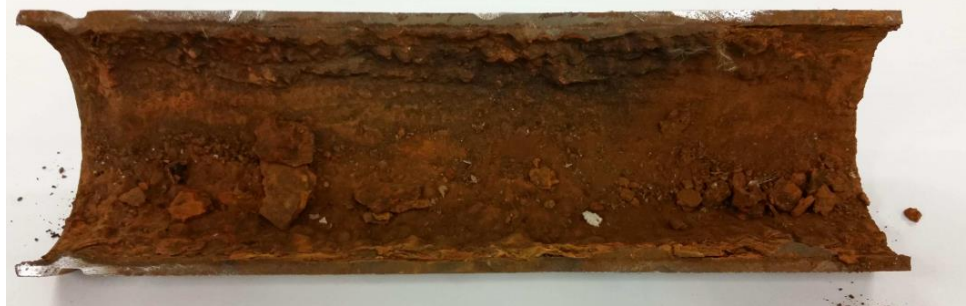
Figure 2: 3" Horizontal Galvanized Steel Domestic Cold Water Pipe
