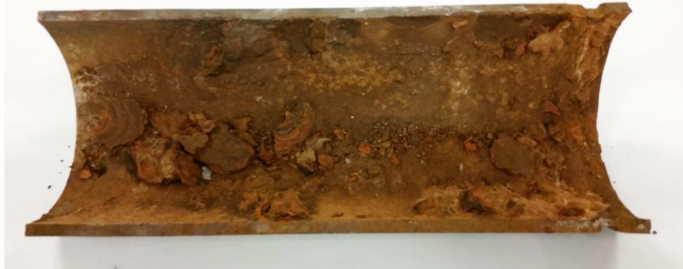
Figure 1: 4" Horizontal Galvanized Steel Domestic Cold Water Pipe
